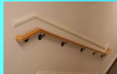
Figure 5. Handrail should extend beyond stairs and be properly attached to the wall.
